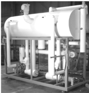
Ammonia Recirculation System
