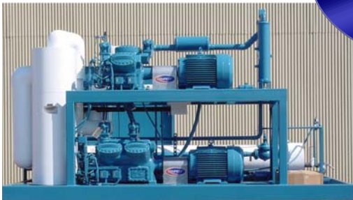
Two Stage Low Temperature Chiller System
